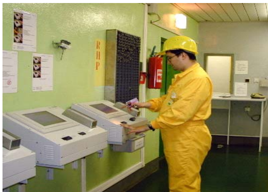
Picture 2: Arrangement of data stations of Electronic Personal Dosimetry System
