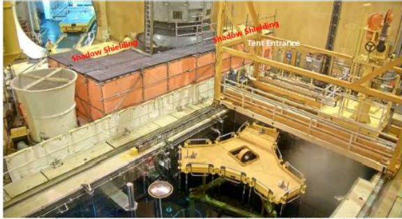
Overview of tent showing tent entrance and extent of tent roof "shadow shielding"
