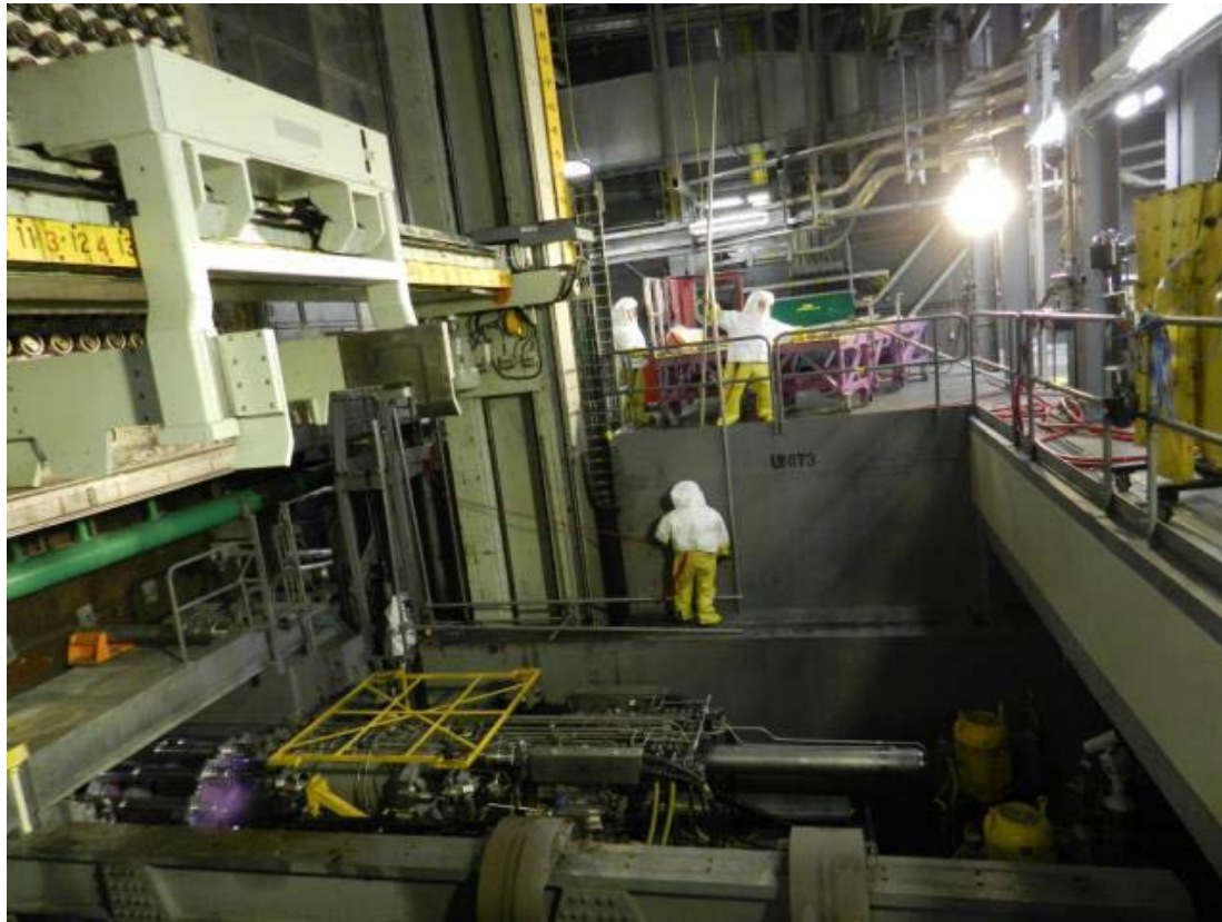
Opening to Duct Requiring Bulkhead
