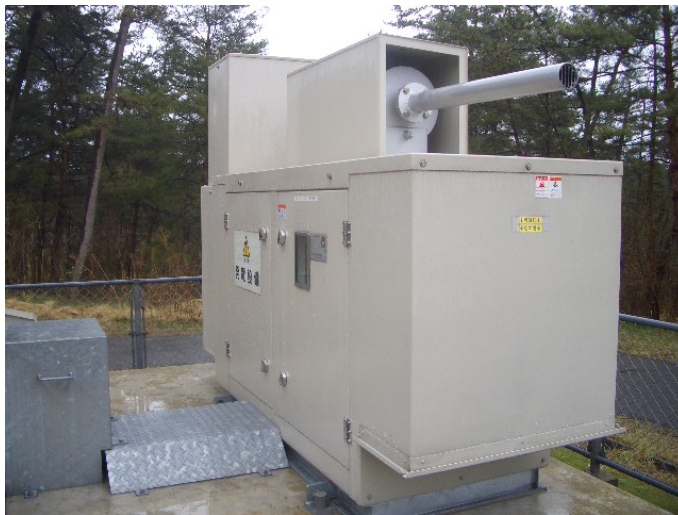
Generator to backup power supply to monitoring posts
