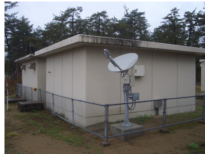
Satellite antenna for monitoring posts
